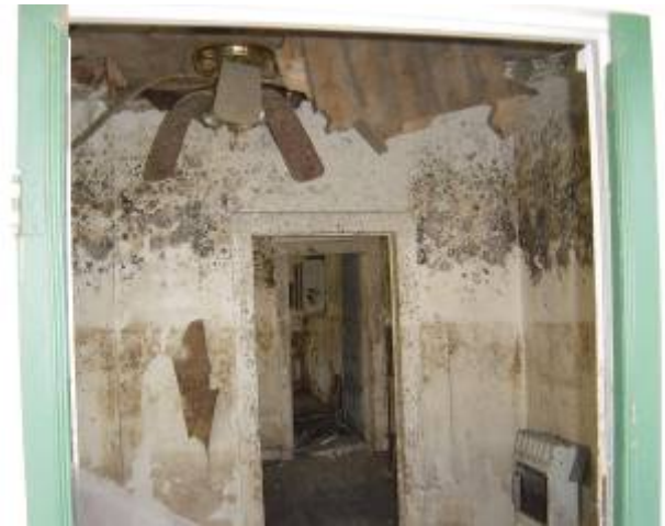
Water-damaged New Orleans home with extensive mold growth, March 2006.
